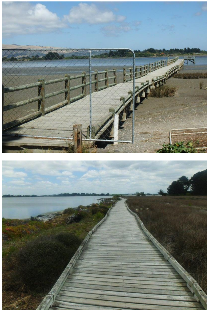
Figure 5: Damage to the jetty and boardwalk
